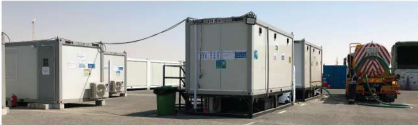
Acid Gas Removal Plant (AGRP)
